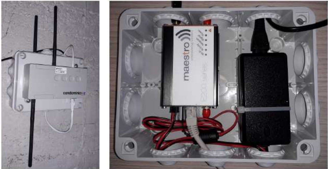
Figure 9: Installation inside a specialized personnel only area on the cover of small wall mount enclosure
