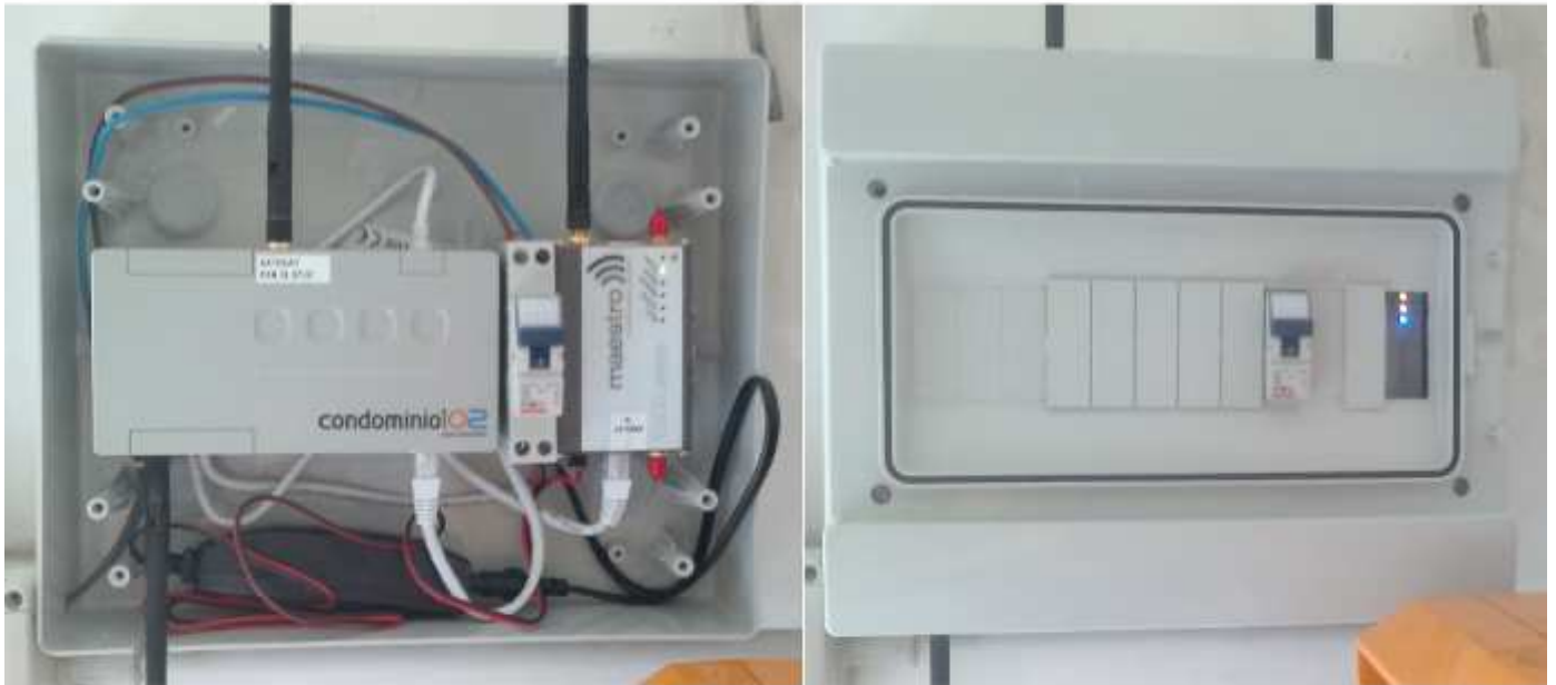
Figure 8: Installation inside an electrical wall mount enclosure
